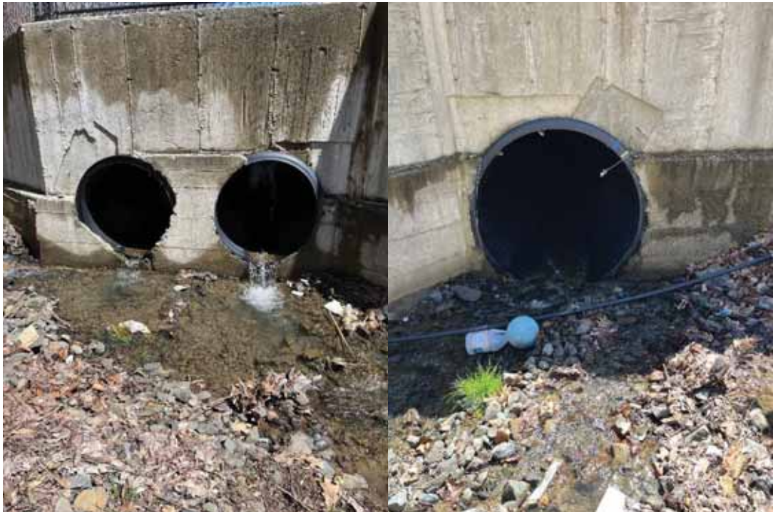
Photos 2 (Left) and 3 (Right) – Stream A culverts facing northeast (Left) and east (Right).
