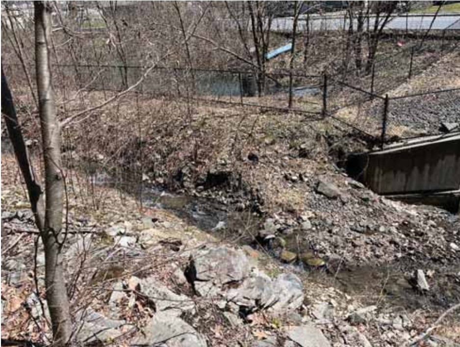
Photo 1 – Stream A (Intermittent Stream/Ditch/Artificial Intermittent Stream) facing northeast, view of Karlsburg Road in the background.
